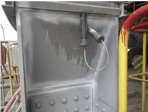
Fig. 4. Cracking at the weld in the tower supporting structure
